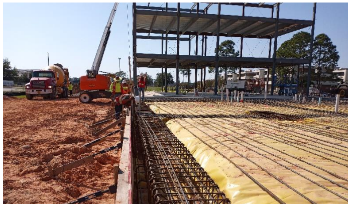
Steel erection started at the west end of the building prior to the completion of the foundation slab for the total structure.
