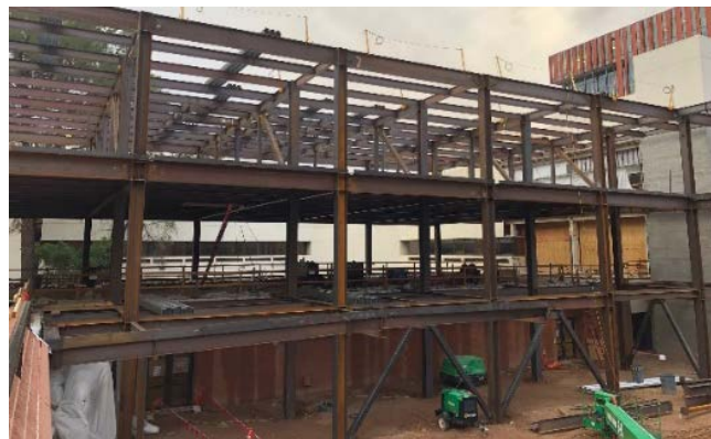
New steel braced frames at the first level and moment frames at levels 2 to 3 and 3 to roof.
